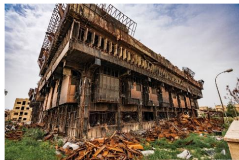
Photo: a damaged building of the Technical University of Mosul (© UNMAS)
